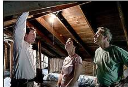
At Susan and David Gaines's home in Arlington, Justin Aruck of EMO Energy Solutions describes how heat is being trapped in the attic. Aruck offered improvement tips. (By Michael Williamson -- The Washington Post)
